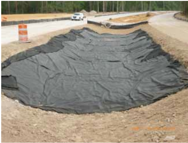
Figure 28: Protected FocalPoint Biofiltration System
