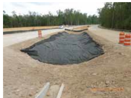
Figure 32: Protected FocalPoint Biofiltration System
