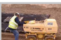
Fig. 23 Vibratory compaction of side backfill is ALWAYS REQUIRED, regardless of what backfill material is used.
