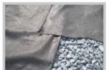
Fig. 6 Reduced overlaps don't create significant savings and can create delays.
