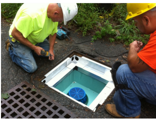
Typical MS4 catch basin draining to Lake Oscawana
