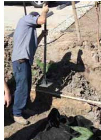
Figure 19: Compaction is critical in order to keep soils from settling around the tank.
