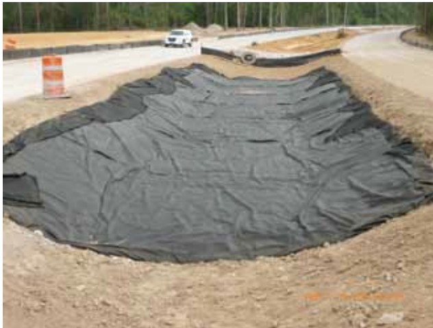
Figure 28: Protected FocalPoint Biofiltration System
